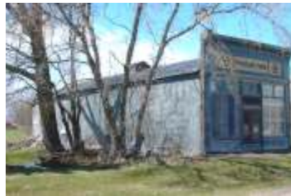
New steel roof on the cash store and corner facial piece reattached by the Bolin Brothers during April for owners Wanda and Richard Melchert.
