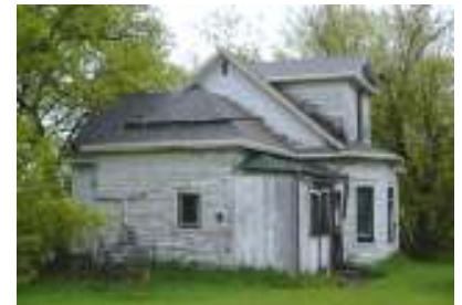
New roof nearing completion on the Johnson-Ostrem House by Greg Seidel and crew during May for owner Rod Anderson.
